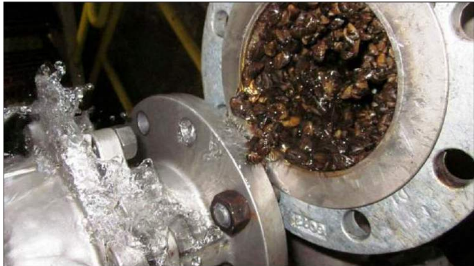
Figure 2: Zebra Mussels Clogging a Pipe
